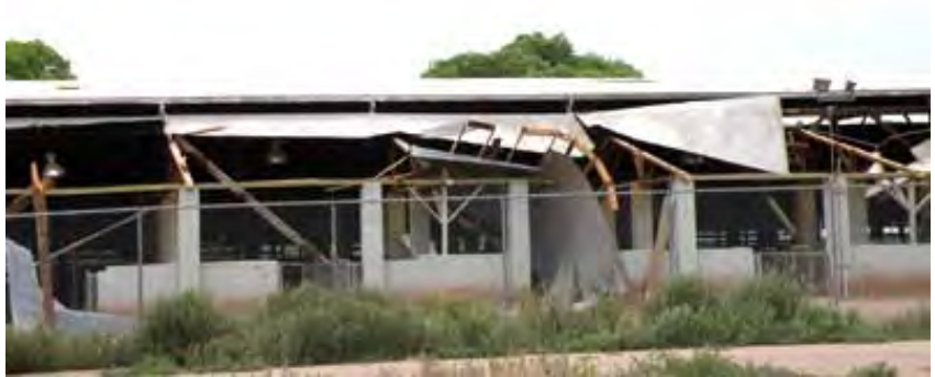
Wind damage, County Fairgrounds, 2012
